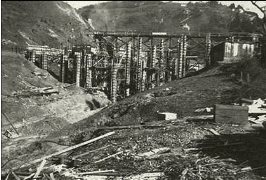
Figure 16 – UC Berkeley Memorial Stadium under construction, 1923 Note concrete culvert. (BAHA archives, courtesy of R. Wesell)
