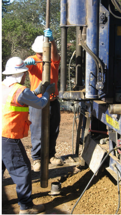
Photograph 3: View of crew members removing casing containing sample from BL 35, facing west
