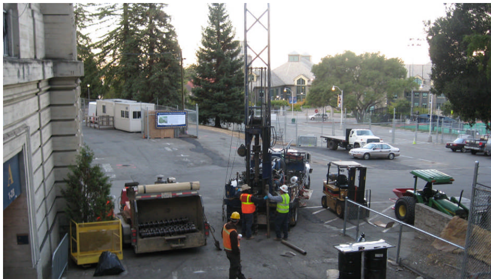
Photograph 8: View from stairs near northwest entrance showing drilling of BL 2, facing southwest
